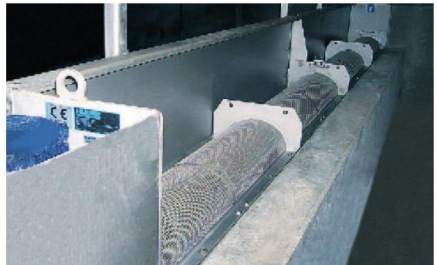
HUBER Storm Screen ROTAMAT® RoK2 installed on foul side of overflow weir
