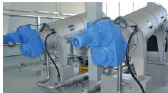
Two HUBER Screw Press Q-PRESS® units installed in parallel
