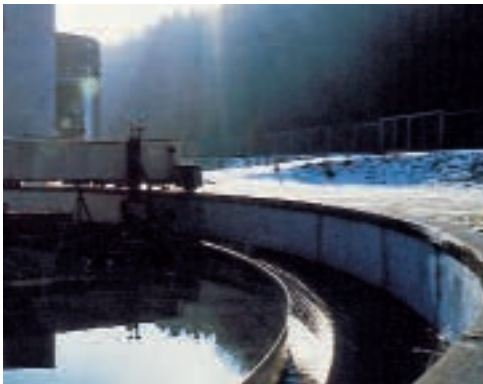
Optimized clarifier equipment
