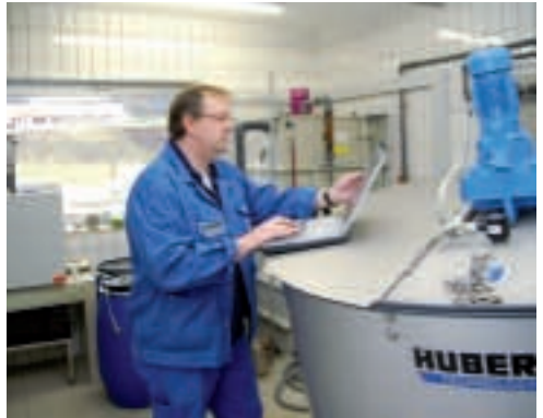
HUBER maintenance service
