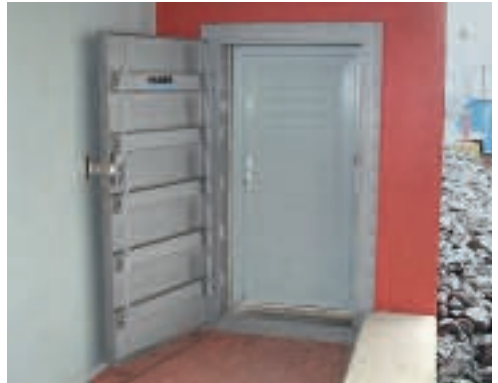
Pressure door installed for flood protection
