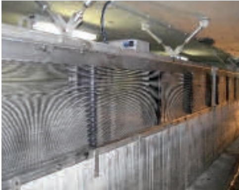
HSW Screen installed vertically on top of the overflow weir
