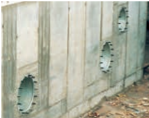
Flush with the wall
